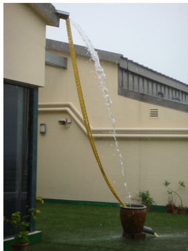
Figure 3.4: Rain in the terrace
